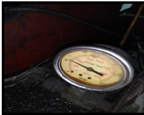
Gambar 16. Tekanan pressure gauge
